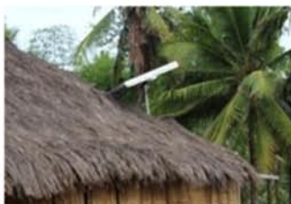
Solar Home System
